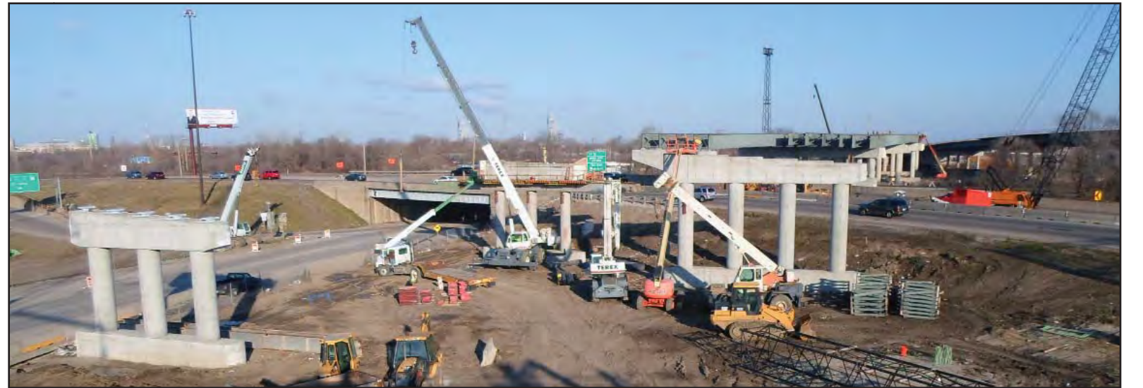
An on-the-ground look at the new ramps from the Tri-level interchange to the relocated I-70.
