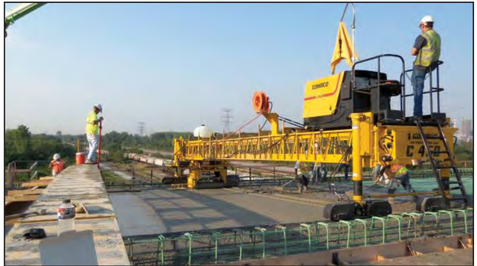
Workers construct the driving surface of one of the many bridges being built to connect the Tri-Level Interchange with the new Mississippi River Bridge.
